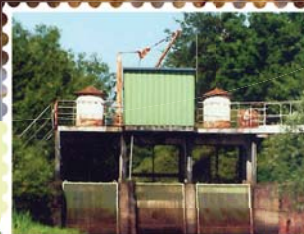
Station de pompage (Mazerolles)
